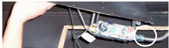
Gas Inlet Line
