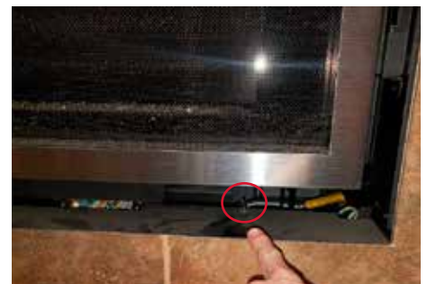
This Surefire switch is located at the bottom right center, behind the front wall.
