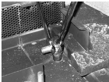
Burner Orifice Removal
