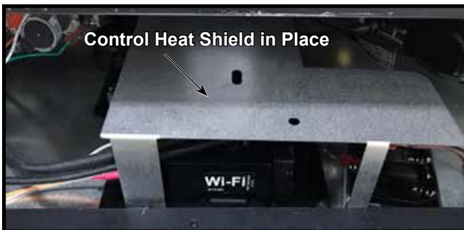
Figure 11.2 Control Heat Shield - Installed
