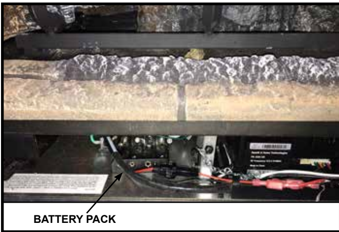
Figure 6.3 Battery Pack Installed
